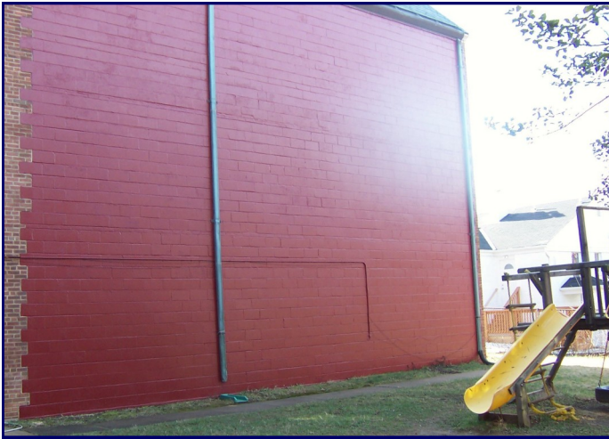
Cracks in our back wall have been sealed and the whole wall has been waterproofed and painted.
